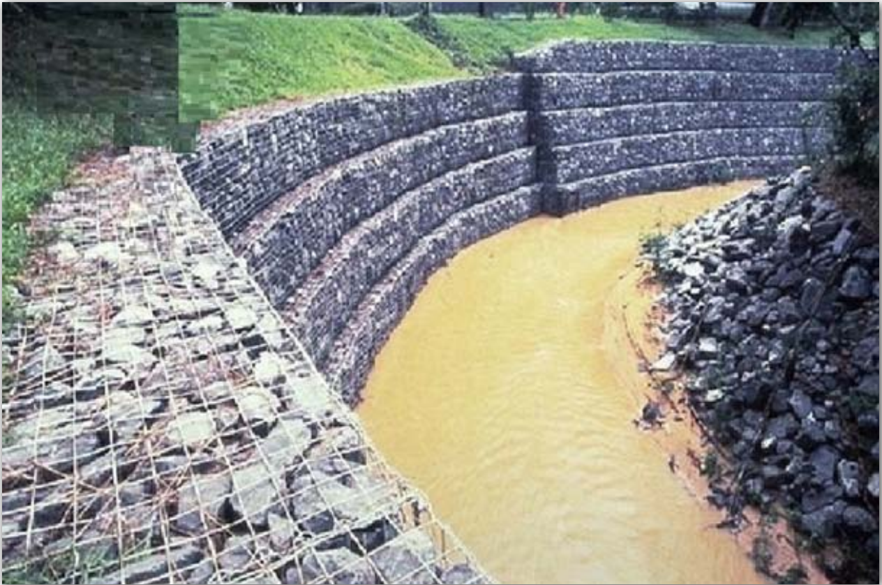
Fig 10.7 Gabion basket placed at river bend to prevent river bank erosion during flooding
